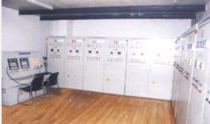
Central control room of distributed control system
